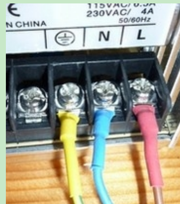
Mains wires in position
